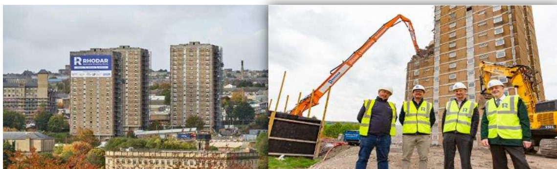
Figure 11 Beech Hill Halifax. Demolition of empty tower blocks and development of 100 homes will make a significant contribution to housing delivery.
