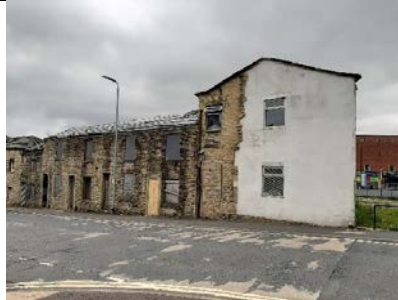
Dilapidated buildings Hopwood Lane
